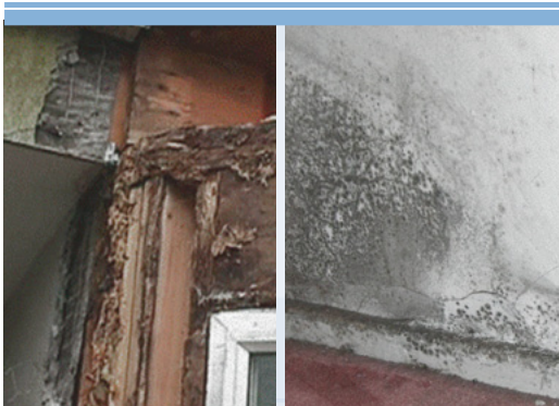
Left: Moisture damage Right: Mold growth
